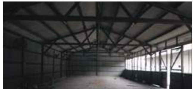
This old shoe factory was constructed using huge quantities of Malaysian hardwood including chengal
